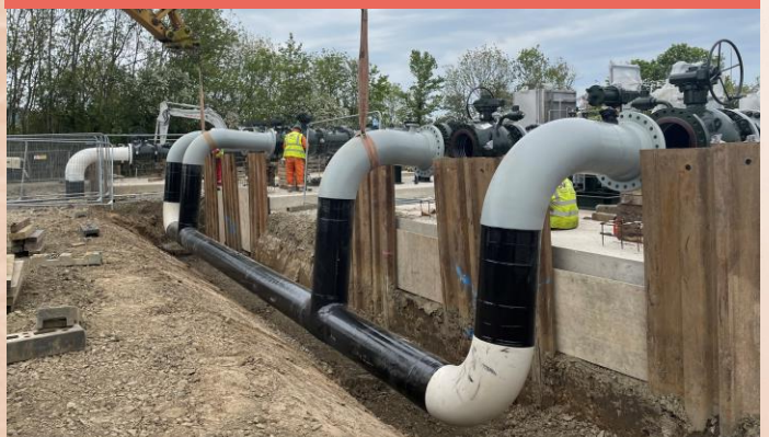
Belowground Pipework Supplying AGI
