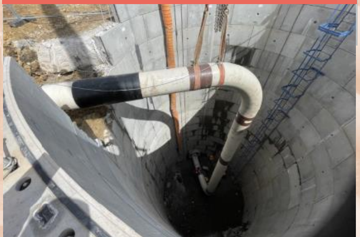
Pipework from Microtunnel Connecting AGIs North & South
